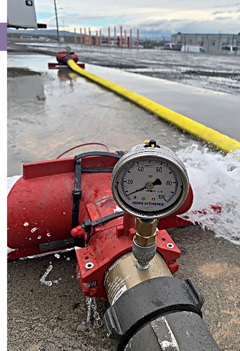
Water flows during CPCCo Soil & Groundwater Shop dry riser system flush.
