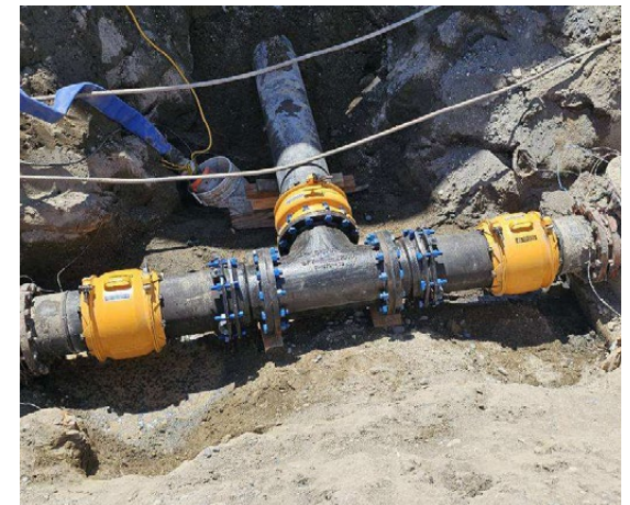
Teams installed new equipment to fix a leak affecting drinking water at the Canister Storage Building and 2704 HV ("Smurf").
