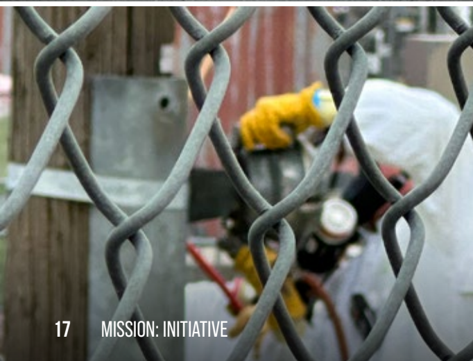
Electrical Utilities crews repair and replace wooden poles as part of a large Sitewide project.
