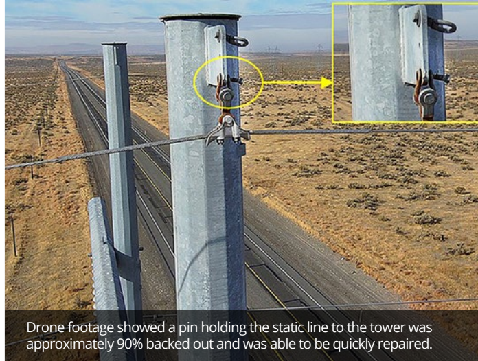
Drones provide a comprehensive aerial view of electrical infrastructure, streamlining inspections and improving damage detection.
