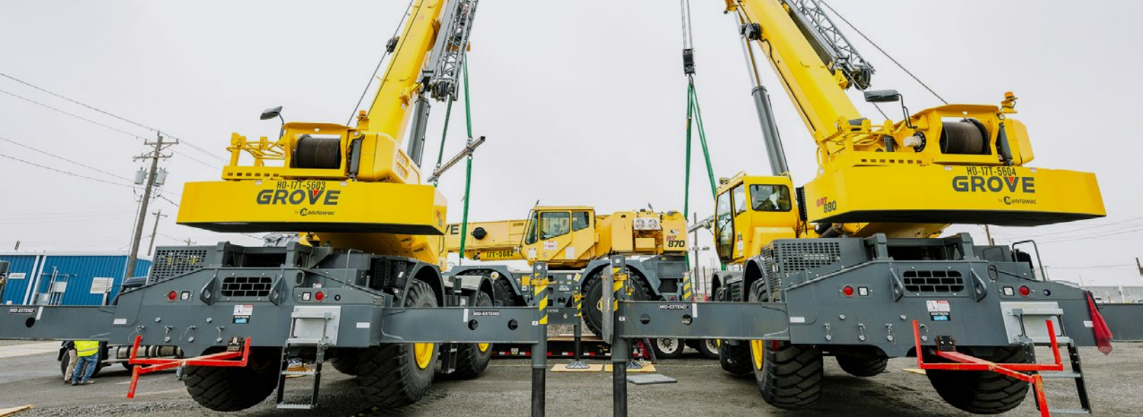
With the combined strength of two 80-ton cranes, the disabled crane is successfully loaded onto the trailer.
