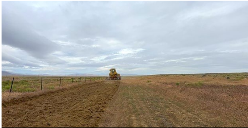
The Hanford Fire Department Fuels Group successfully completed a 33-mile fire break disc line to minimize wildland fire risk to the Hanford Site.
