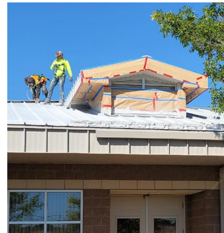
Subcontractor workers add a membrane coating to the Administration Building on the campus of the HAMMER Federal Training Center.
