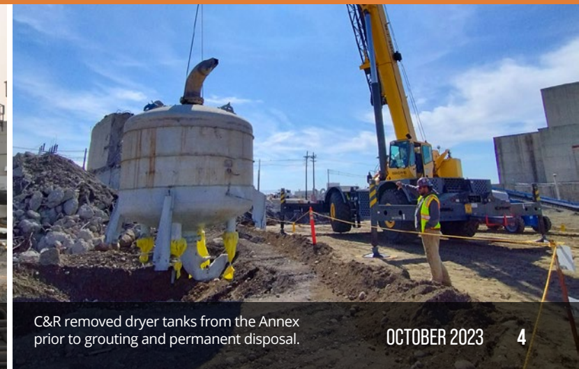
Crane & Rigging crews removed the roof of the K West Annex as part of its demolition.
