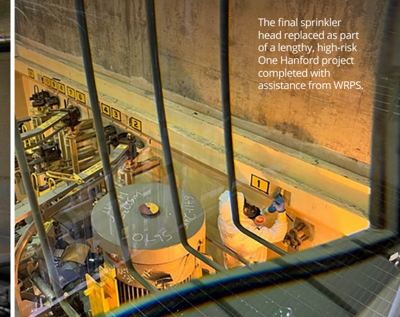
Crane & Rigging crews built scaffolding to allow our Fire Systems Maintenance team to access high elevation sprinklers in the 242-A Evaporator.
