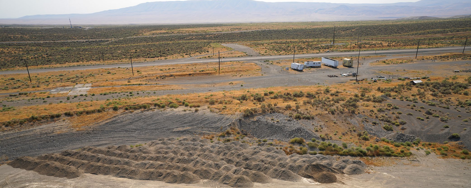
An aerial view of the mounds of material from the Effluent Treatment Facility construction project currently stored inside Pit 30. The material will be used for other construction and remediation projects around the Hanford Site.
